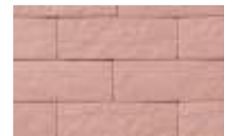
BK-1204 without grouting
