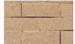
BK-1203 without grouting
