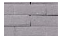
BK-1305 without grouting
